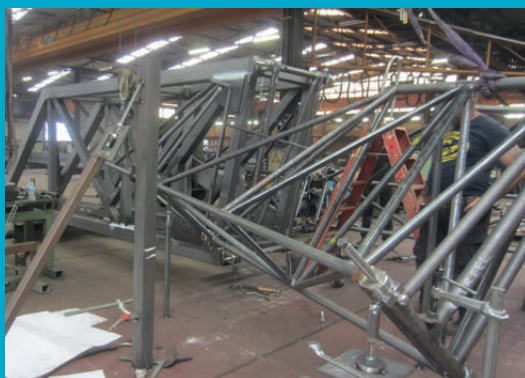
▲ The cross vault of the Bravo structure made for some extremely complex steel joints.
